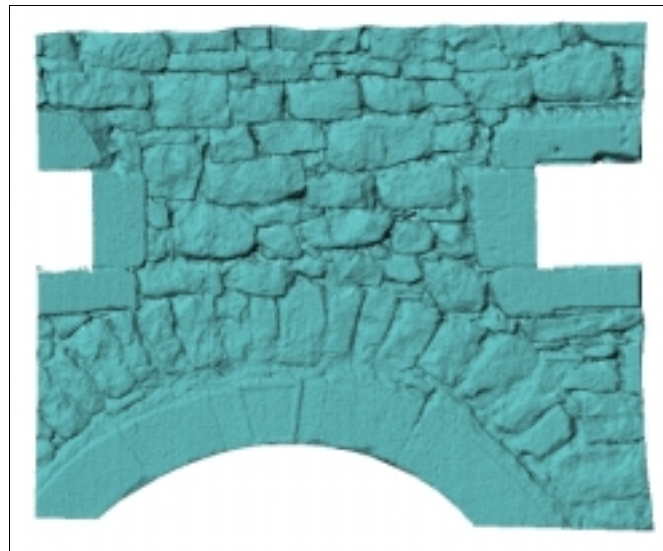
Figure 10: Detail of a ruin wall (without texture) containing quarry stones and cut stones. Size about 2.3 m x 1.8 m.
